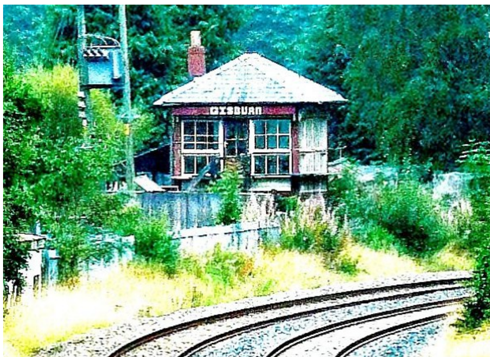
The privately-owned signal box at Gisburn still stands but, having viewed it from the Ribble Valley Rambler services, its condition appears to be deteriorating
